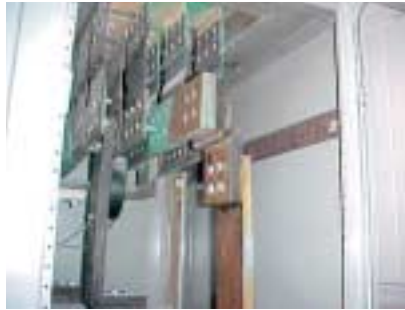
Even though load readings and a visual inspection did not indicate a problem, the infrared readings (below) revealed a problem with the buss section.
